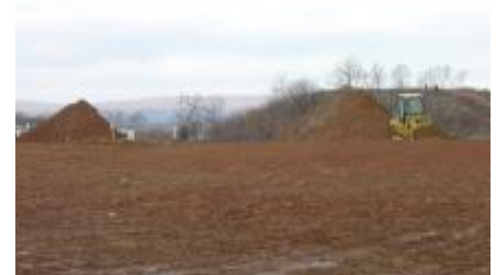
The new parking lot adjacent to the Purcellville Facility is expected to be completed in early 2006.
